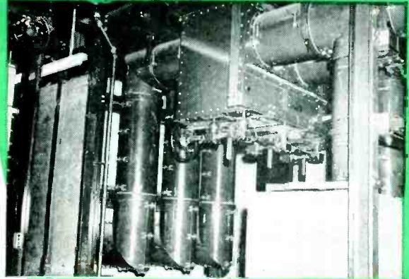
A completed portion of metal enclosed bus and switches shows how neat and compact the 3500 Ampere Isolated Phase Bus installation is at Consolidated Edison's Waterside No. 1 station.
